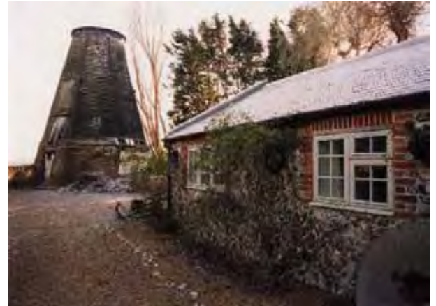
The smock mill is in urgent need of repairs
