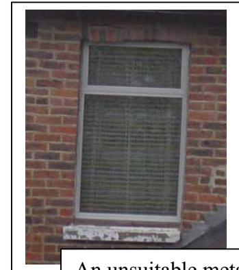
An unsuitable metal window
