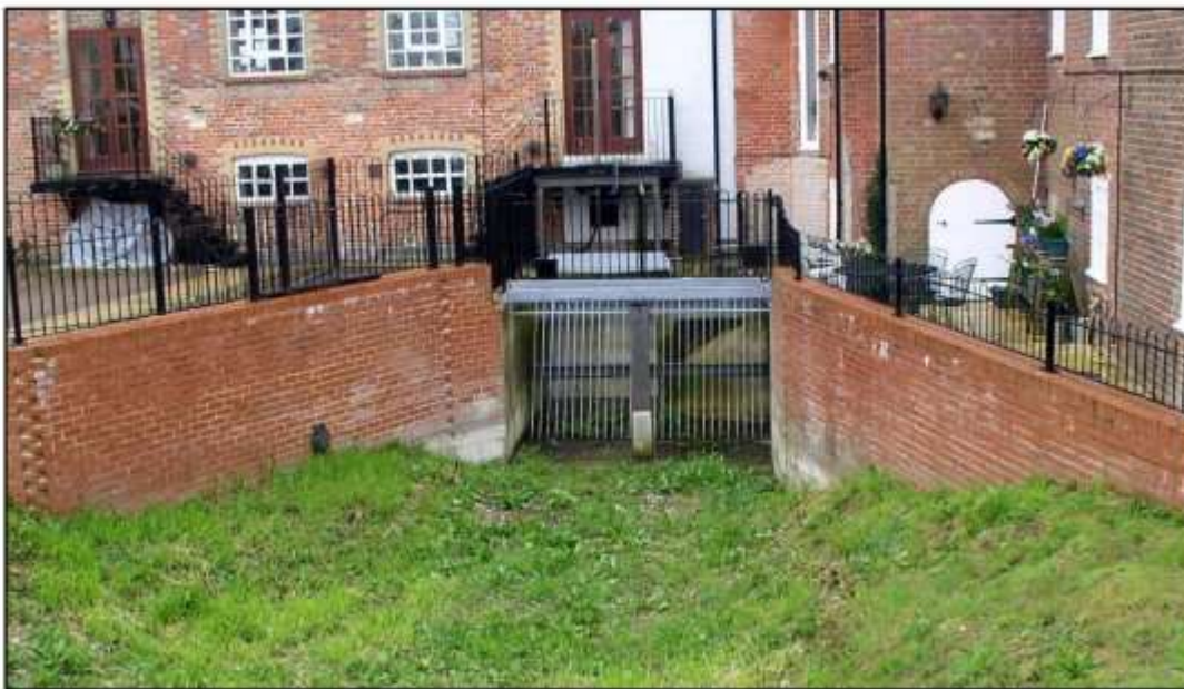
Figure 2-3: Penstock at Westhampnett Mill
