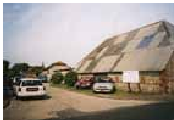
The listed barn needs a new roof
