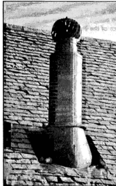
An unsightly metal flue
